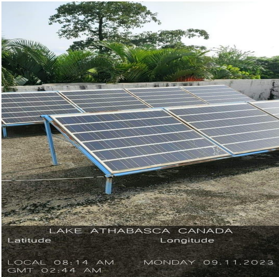
Solar Cells at Library Building
