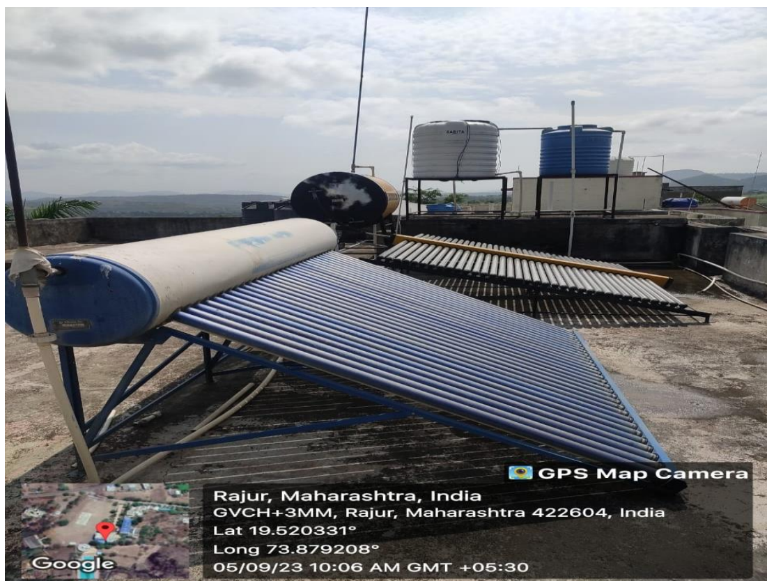
Solar Water Heater at Ladies Hostel
