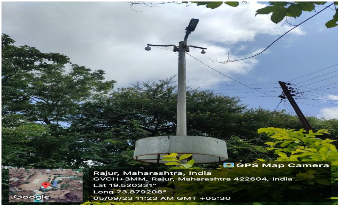
Solar Street Light
