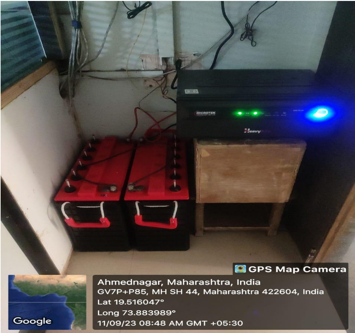
Uninterrupted Power Supply
