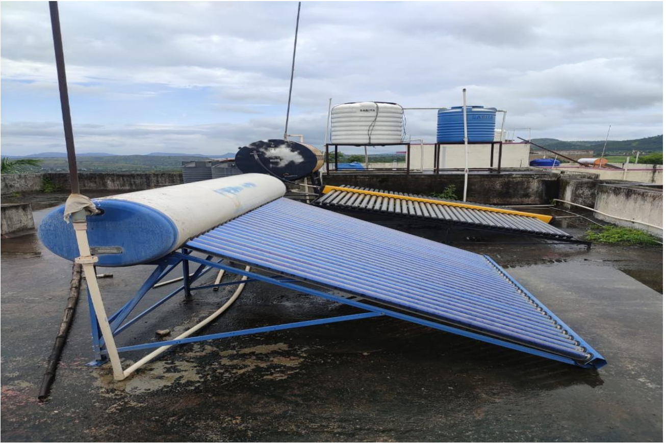
Hot Water System
